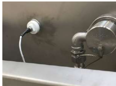
Valve shown mounted on mixer. Temperature sensor shown to the left and valve shown to the right.
