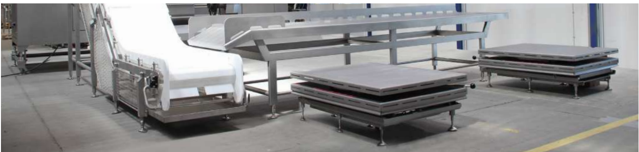
Belt Conveyor with unpacking station with 2 (two) lifting tables for ergonomics, left side.
