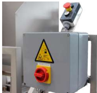
Operator/control panel with emergency stop.
