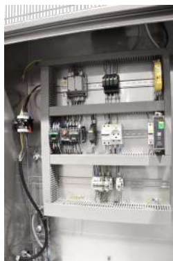
View inside electrical panel.
