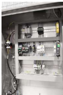
View inside electrical panel.
